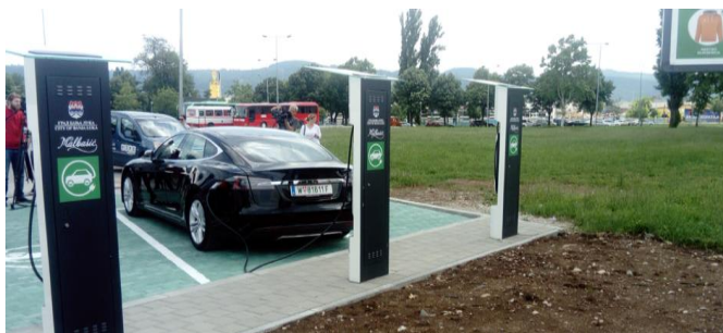
Figure 3. Chargers for electrical vehicles
