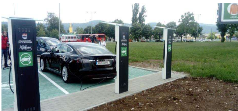
Figure 3. Chargers for electrical vehicles
