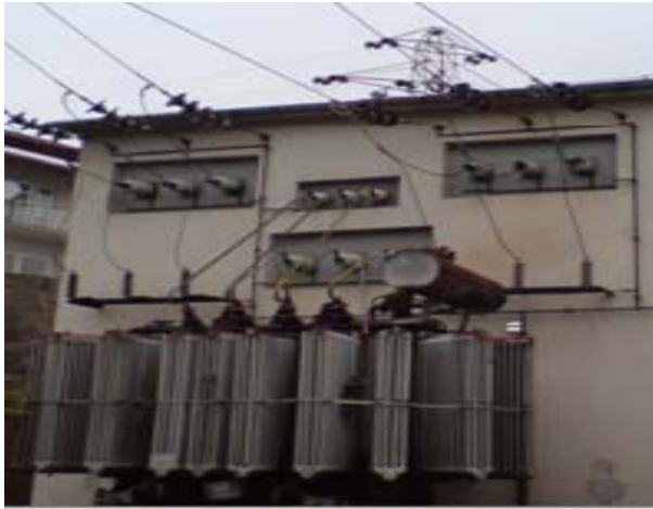
Fig. 2. A transformer installed in a power grid in a substation [3]
