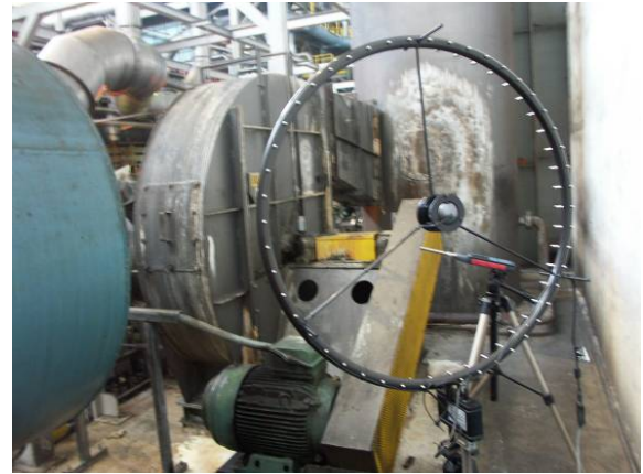
Fig. 8. Installed Acoustic Camera by exhaust plant.
