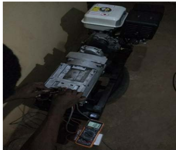
Fig. 9. Voltage testing of the alternator/generator
