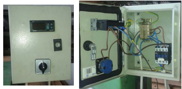
Fig. 14. Electrobox with electrical components
